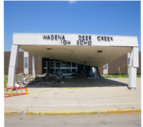
Tornado damaged building
