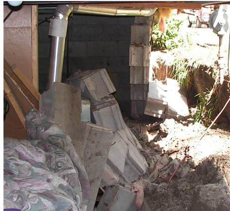
Flood damaged building
